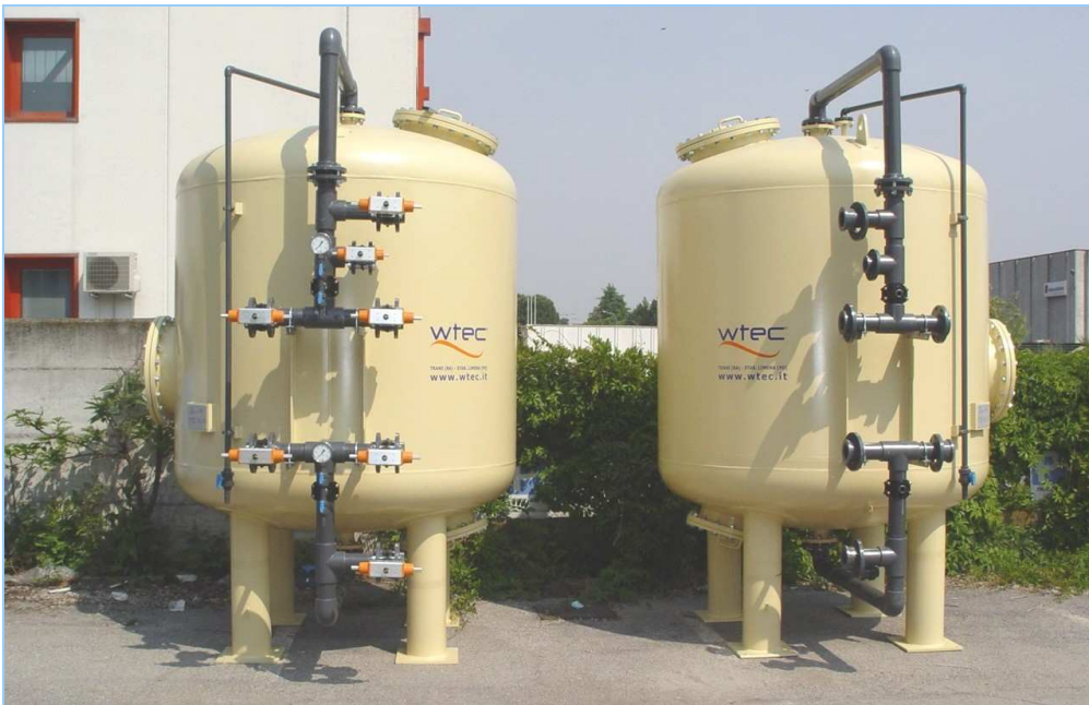
Pretrattamento Osmosi Inversa - Reverse Osmosis Pre-Treatment
